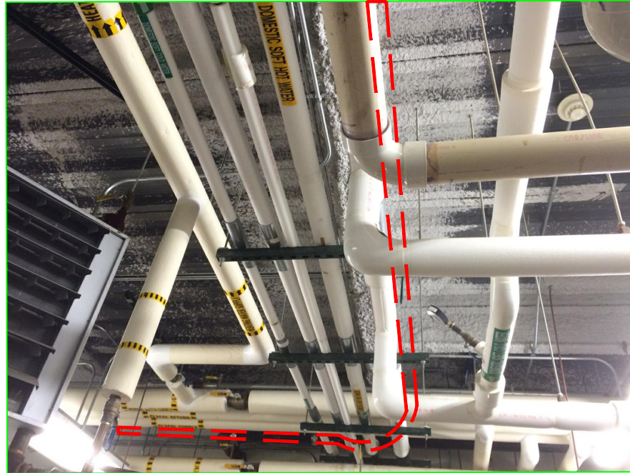
ROUTING ACROSS CEILING
