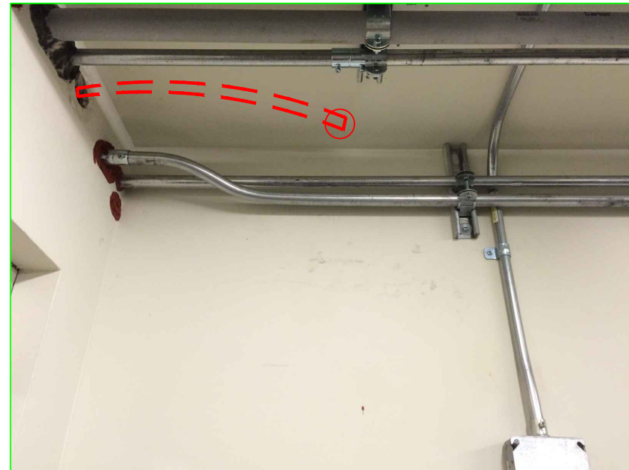
ROUTING FROM WORKOUT ROOM INTO SERVER ROOM SECONDARY AREA THEN ROUTING BACK TO MAIN SERVER ROOM LOCATION
