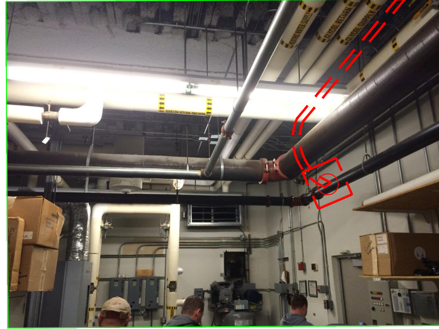
ROUTING ACROSS CEILING TO ROOM EXIT INTO FALSE CEILING
