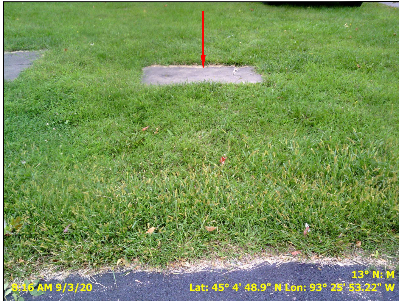
Existing Handhole Windstream
