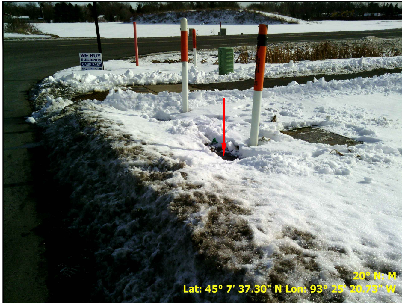
Existing Zayo Vault
