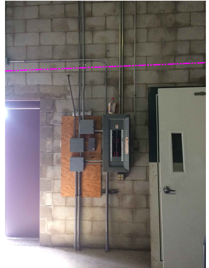
2" EMT ROUTE CONTINUING ALONG WEST WALL. CIRCUIT BREAKER PANEL LOCATION FOR OUTLET FEED.
