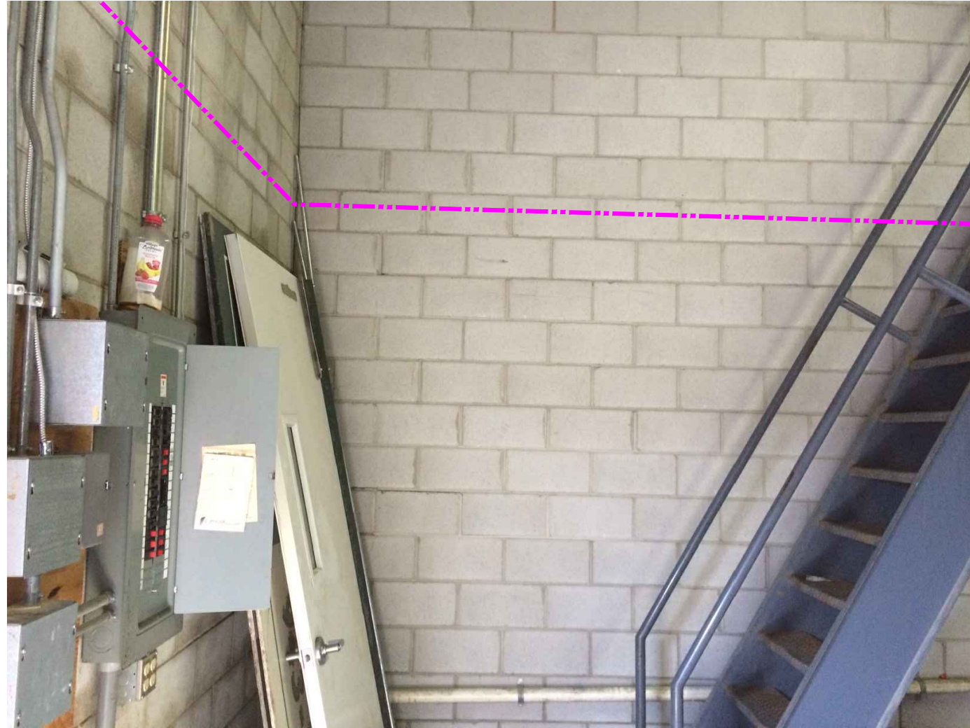
2" EMT ROUTE CONTINUING ALONG WEST WALL AND TURNING ALONG THE NORTH WALL, PAST THE STAIR CASE. CIRCUIT BREAKER PANEL LOCATION FOR OUTLET FEED.
